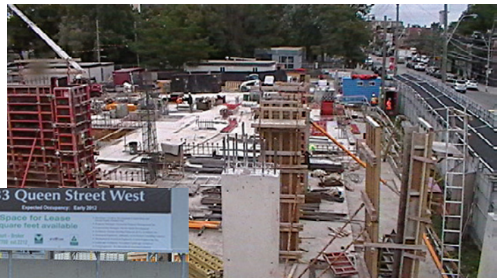
Construction for the first non-CAMH building – the Ossington-Queen Street Rental Apartments – is now above ground.
